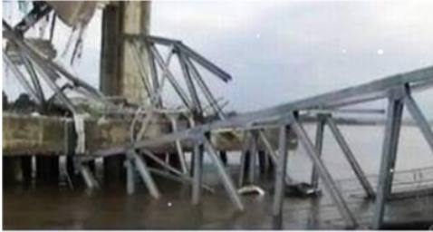
Figure 1. Failure of steel truss bridge
