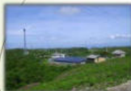
787 kW Solar-Wind-Diesel, Nusa Penida
